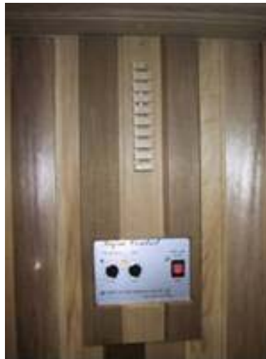
Figure 6 Control Panel Front mounted
