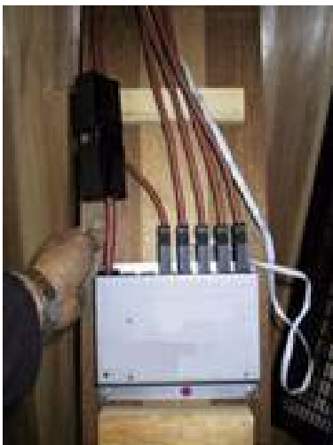
Figure 5 Control Panel rear.
